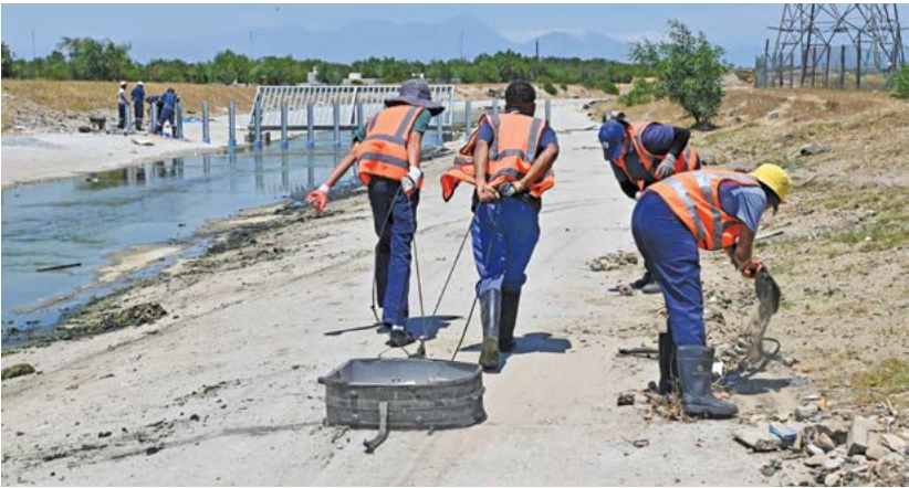
Come on, canal's not a trash can! Boosted waste interceptor capacity in the Kleinvei canal is supporting the City's efforts against illegal dumping in this watercourse.
